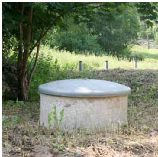
A typical private small scale sewage plant for WC and greywater connected to a three-chambered septic tank with following infiltration. (Source: @avloppsguiden.se)
