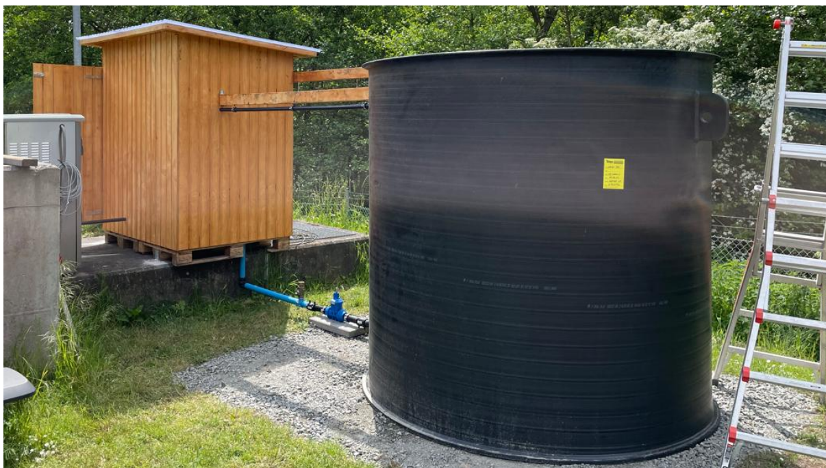
Figure 2: Photo of pilot-scale Slow Sand Filter (SSF) installation at Svaneke WWTP.
