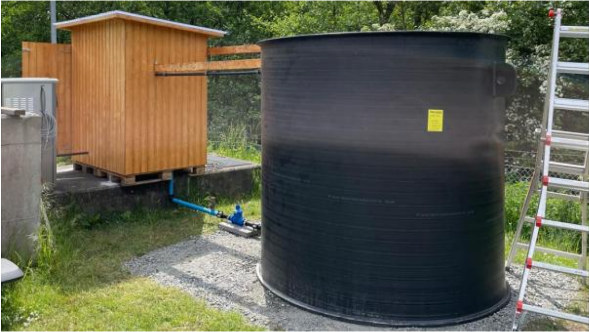
Figure 5 - Photo of pilot-scale Slow Sand Filter (SSF) installation at Svaneke WWTP.
