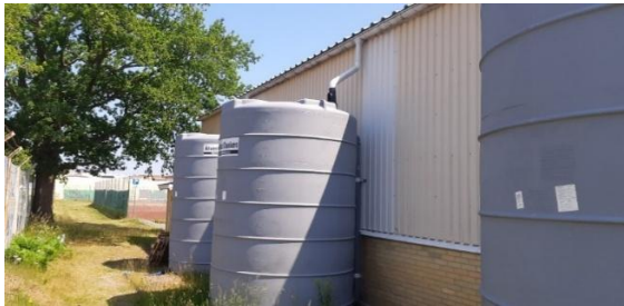
Rain water harvesting Tennis center
